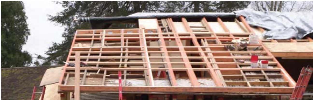
Sistering/structural augmentation complete. The intention of this effort was to stiffen the structure in both directions-similar to an airplane wing.
