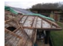
View of hip roof at entry facade replaced with continuous members and the discontinuous valley rafter was replaced with a micro lam.
