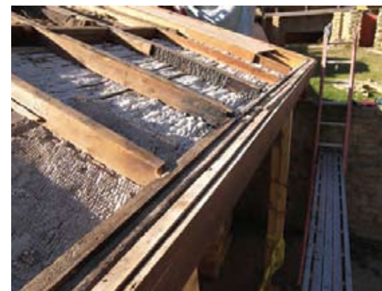
Fire damage to the fascia and rafters.
