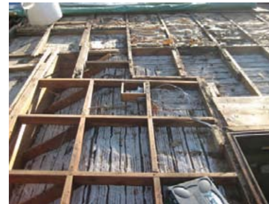
Detail of existing framing. Upper right hand corner shows evidence of an earlier fascia line. This is the right side of the roof shown above- this cantilever was supported by horizontal blocking that resulted in significant failure.
