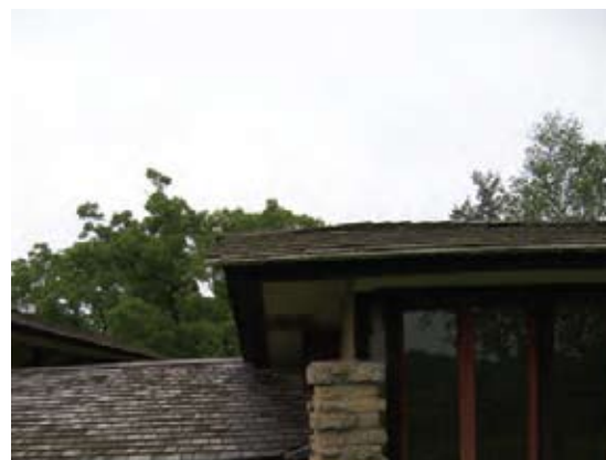
Detail of south eave showing deflection at the extreme ends of the roof structure.
