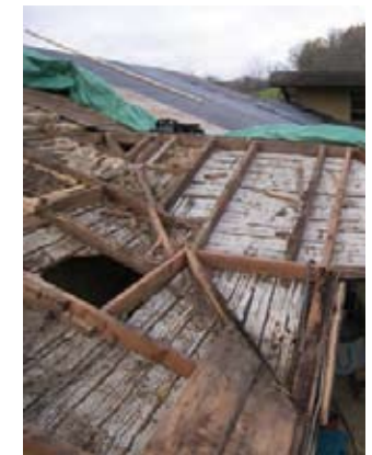
View of hipped roof at entry the f... continuous members and the disc... was replaced with a micro lam.
