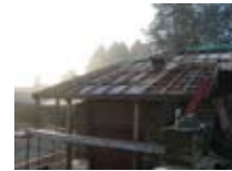
Existing framing condition. The left side of the roof was framed using half lapped notched members to counteract the force of gravity on the overhang.
