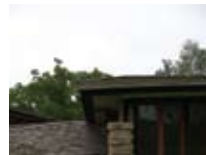
Detail of rafters showing deflection at the extreme ends of the roof structure.
