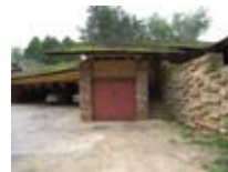
One of the most seriously deflected rafters in need of structural rehabilitation. The above roof cantilevers to the front and side elevations.
