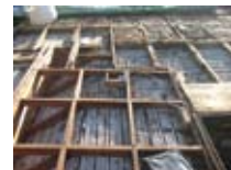
Detail of existing framing. Upper right hand corner shows evidence of an earlier fascia line. This is the right side of the roof shown above. This cantilever was supported by horizontal blocking that resulted in significant failure.
