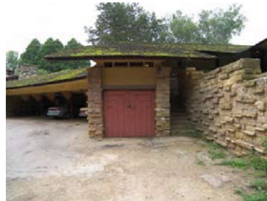
One of the most seriously deflected soffits in need of structural rehabilitation. The above roof cantilevers to the front and side elevations.
