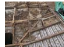
View of the failed valley at the entrance to the West Wing.
