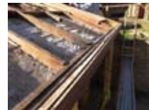
Fire damage to the fascia and rafters.
