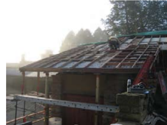
Existing framing condition. The left side of the roof was framed using half lapped notched members to counteract the force of gravity on the overhang.
