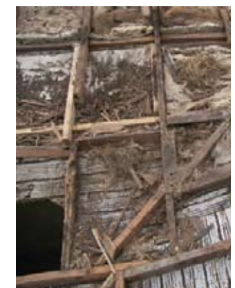
View of the failed valley at the en...
