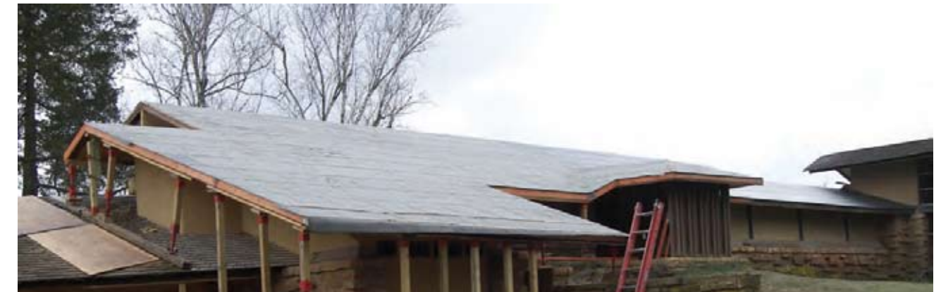
View towards the entrance of the West Wing, all structural repairs have been made, and the roof is ready to receive the cedar shingles.
