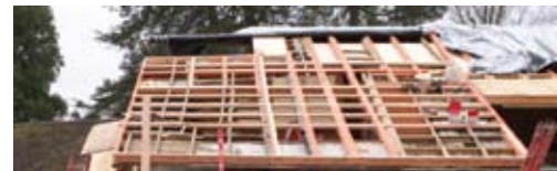
Structural augmentation complete. The intention of this effort was to stiffen the structure in both directions similar to an airplane wing.
