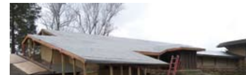
View towards the entrance of the West Wing. All structural repairs have been made, and the roof is ready to receive the cedar shingles.
